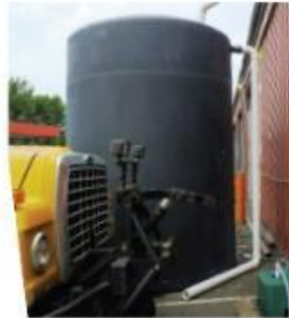
Fig. 1. Five-thousand gallon cistern to collect rainwater and reuse for street sweeping and truck washing at Pamippany-Troy Hills. Department of Public Works facility. Photo credit: Pat Rector.
